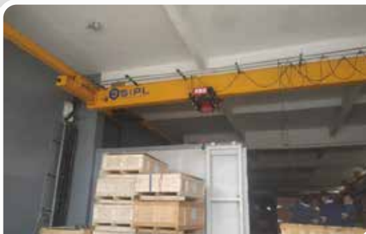
Under slung crane up to 5 ton
